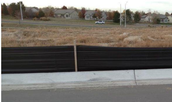
Silt fence with stakes and staples exposed.
