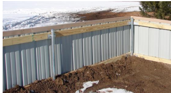
Prairie dog side of barrier. Note safe caps on metal posts and elongated cap along top of metal fencing.
