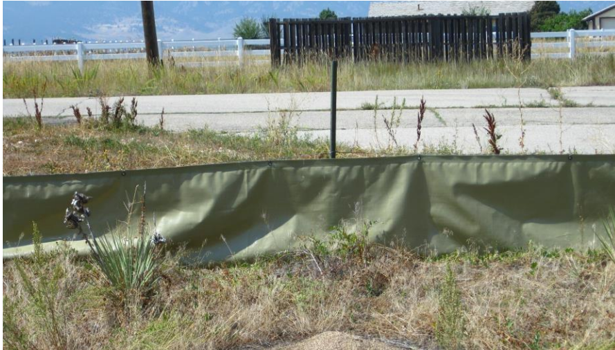
Flawed vinyl barrier installation
