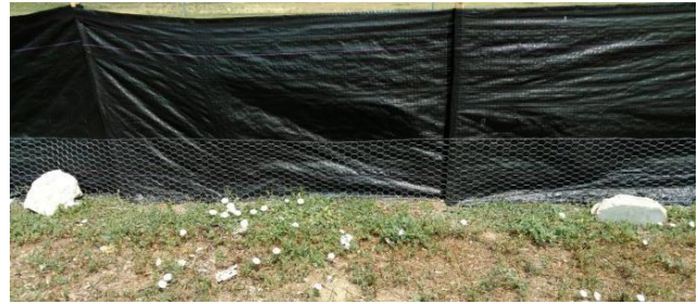
Modification: Using 2 foot-wide one-inch netting poultry wire, lip one foot vertically and use a staple gun to attach to wood posts. Anchor horizontal piece to ground with 6-inch pins.
