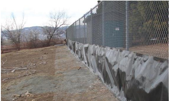
Modified existing chain-link fence to inhibit movement back into park (prairie dog side).
